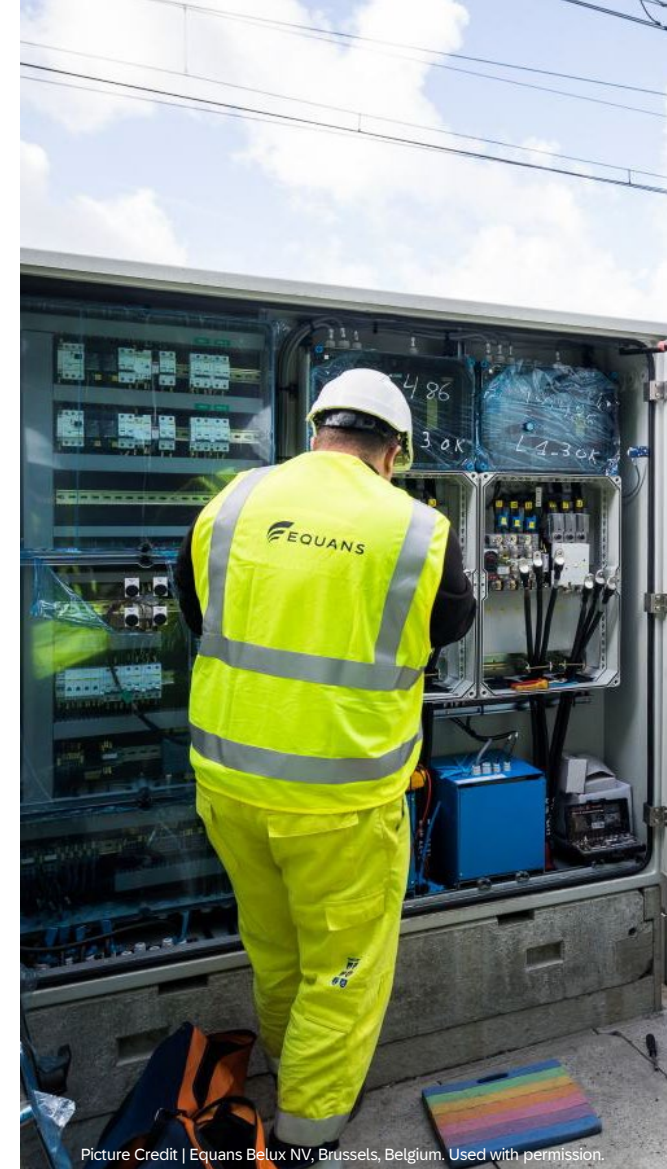
Picture Credit | Equans Belux NV, Brussels, Belgium. Used with permission.
